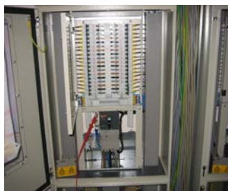
Central Distribution Fuse Panel
