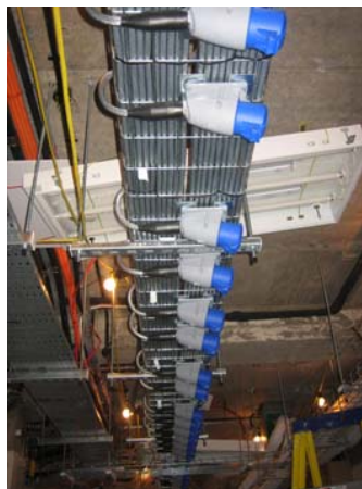
32 Amp Power Outlets
