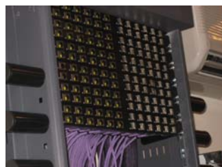
Central Cable Connection Panel
