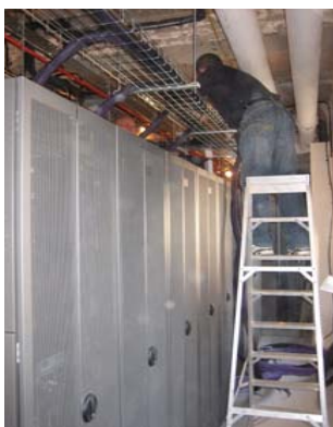
Server Cabinets in Position
