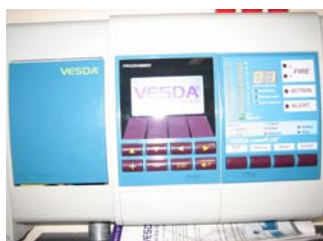
Vesda Smoke Detection Controls
