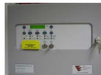
FM200 Gas Controls
