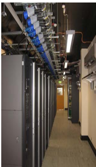
All 17 Server Cabinets in Position
