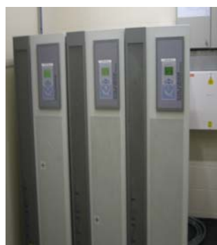
New UPS Room
