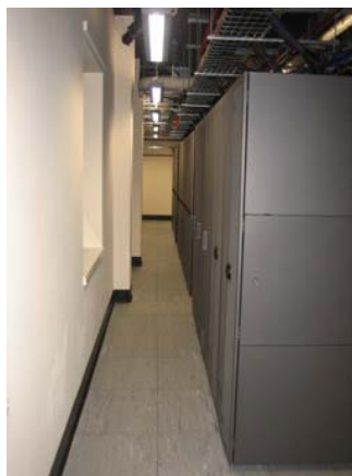
Rear Access to Server Cabinets
